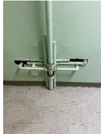
Lavatory drainage piping
