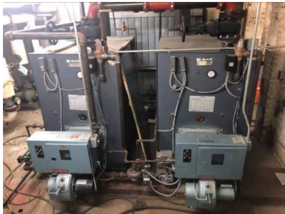
Existing Hot Water Boilers
