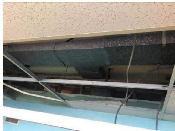
Lower Level- Ductwork
