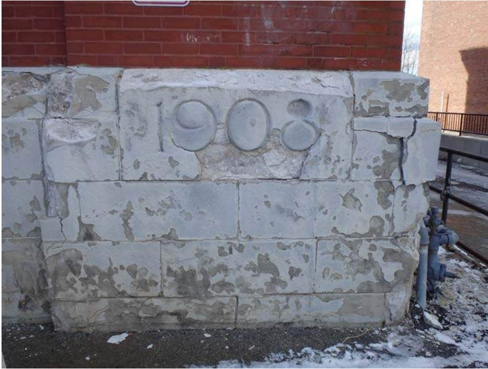
Figure 9. Typical poor condition of foundation cast stone blocks
