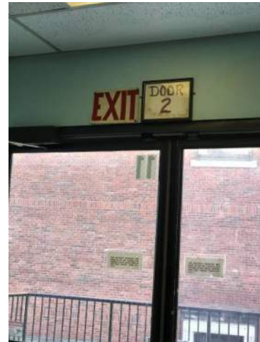
Non-Lit Exit Sign
