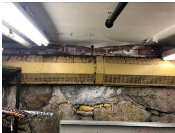
Basement Storage Room – Fin Tube Radiation
