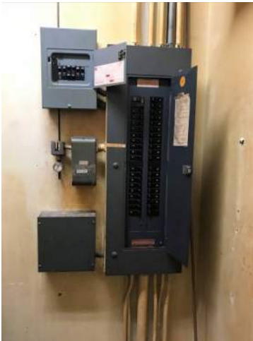
Panelboards with Subpanels
