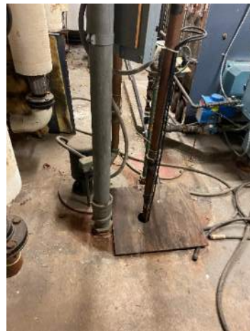
Boiler Room sump pump
