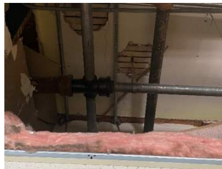
Galvanized vent piping
