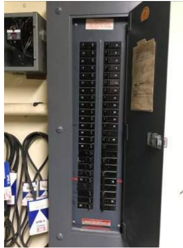
Panel in Basement
