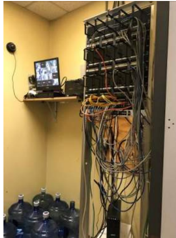
Floor Rack in MDF Room
