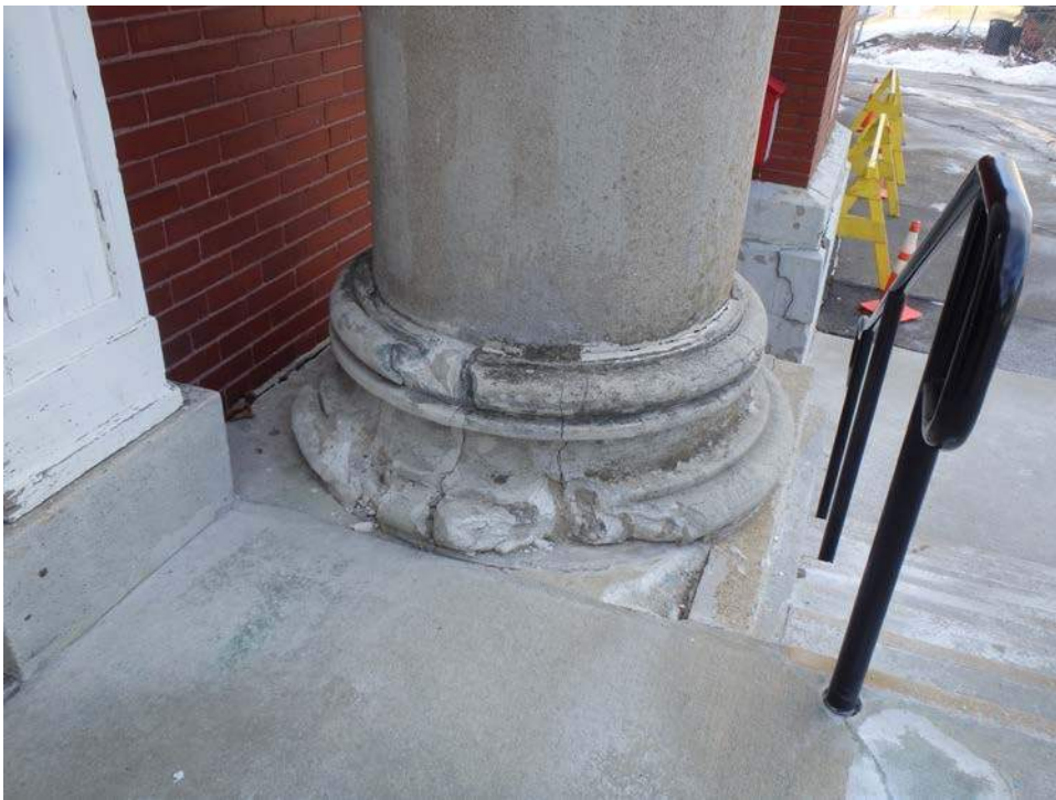
Figure 12. Deteriorated cast stone column base
