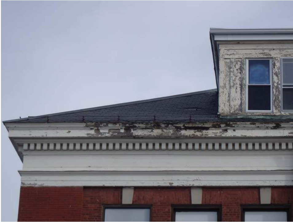
Figure 17. Deteriorated wood at locations where roof water is diverted to cornice
