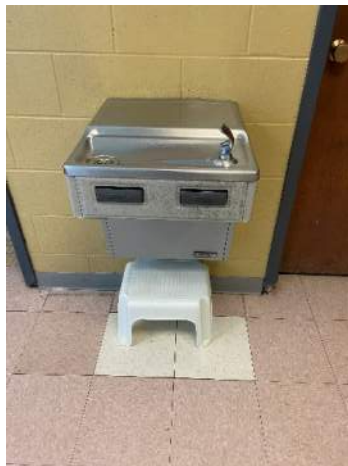
Wall hung water cooler
