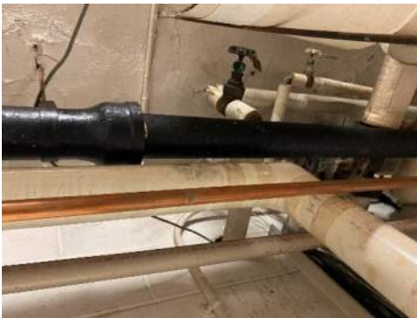
Cast iron waste piping
