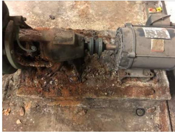
Existing Hot Water Pump P-2
