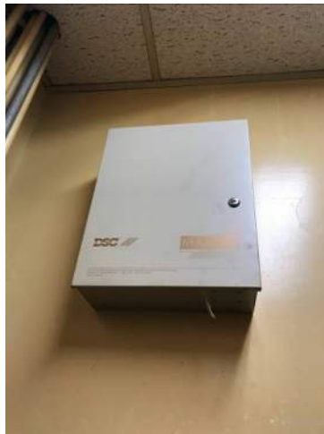
Security Control Panel
