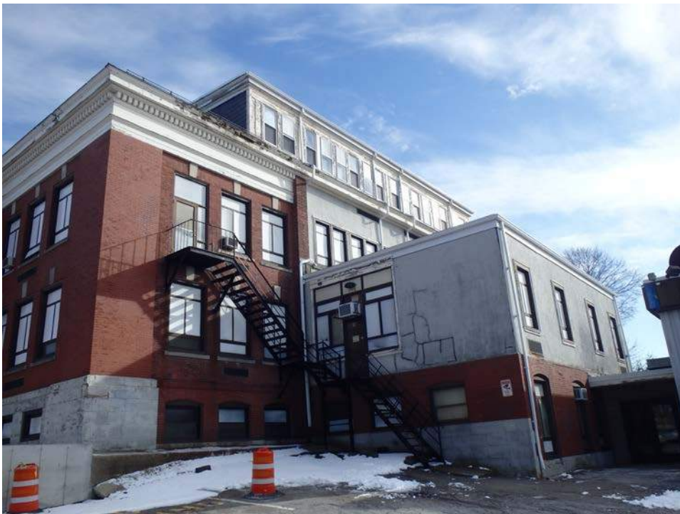
Figure 14. West addition stucco showing cracking
