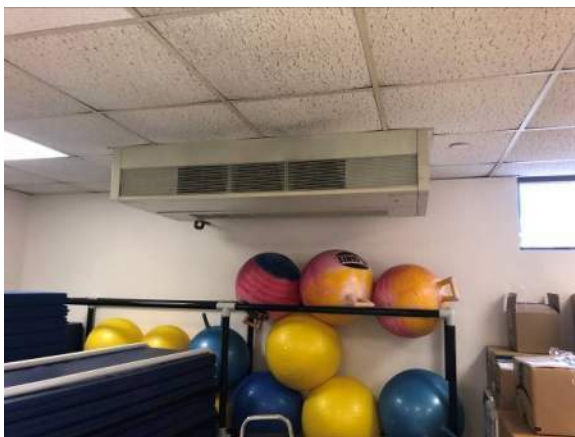
Lower Level- Unit Ventilator
