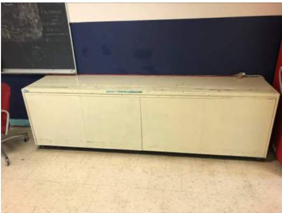
Cafeteria – Unit Ventilator
