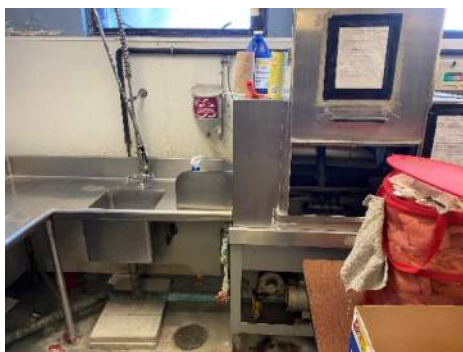
Kitchen pre-rinse sink & dishwasher
