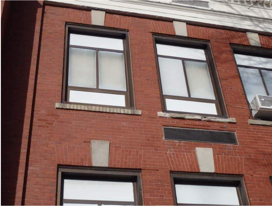
Figure 11. Typical cast stone sill condition (right) and brick rowlock replacement (left)
