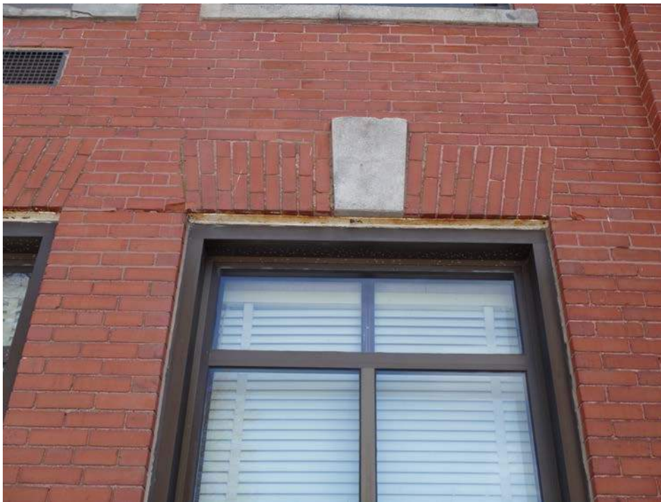
Figure 6. Rusting lintel and spalled brick at edges
