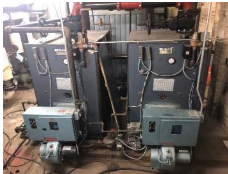
Natural gas supply to Boilers
