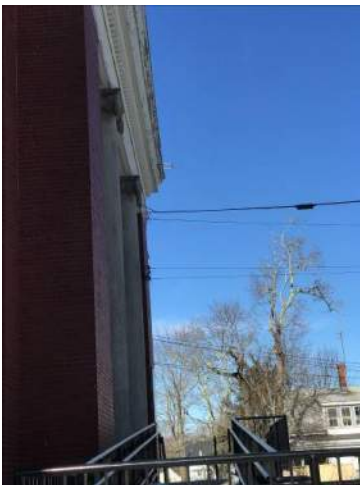
Communications Overhead Services
