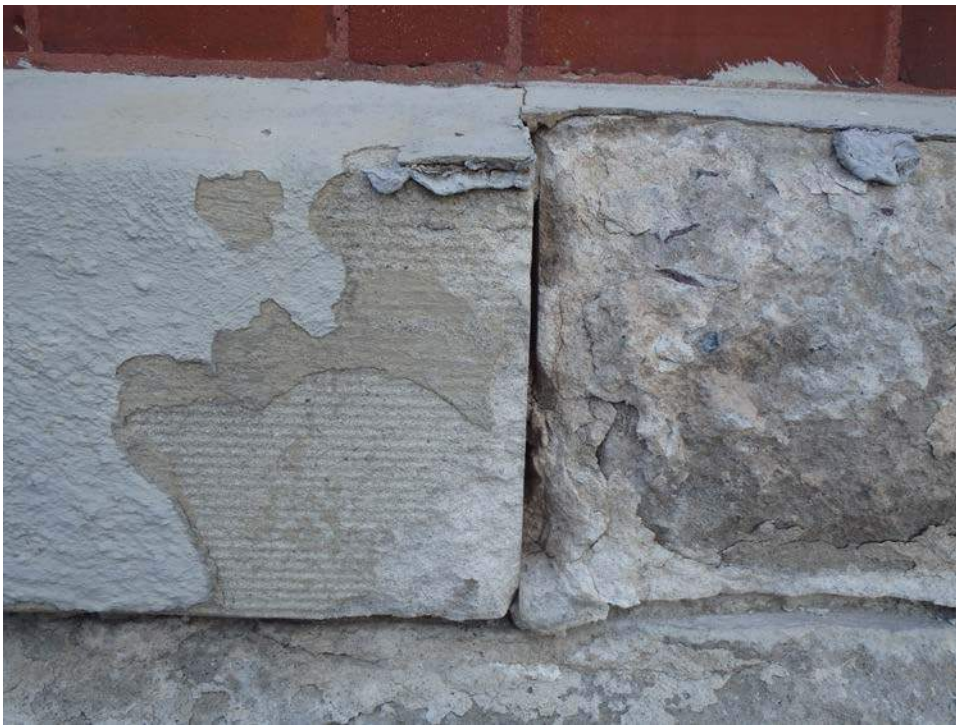
Figure 8. Original cast stone tooling and color exposed under coating
