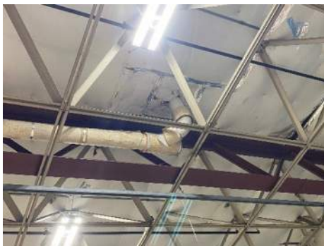
Insulated rain leader piping - Gym
