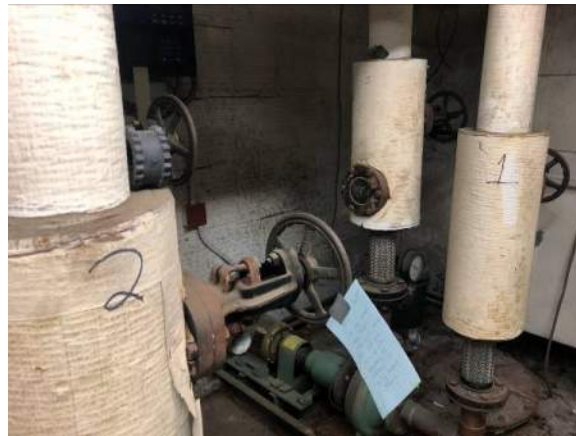
Existing Hot Water Pump P-1
