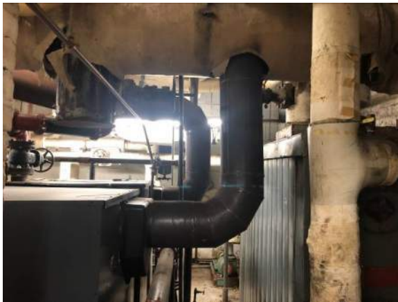
Uninsulated Boiler Breeching
