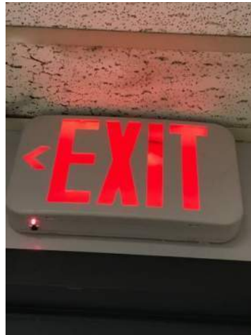
Internally Lit Exit Sign
