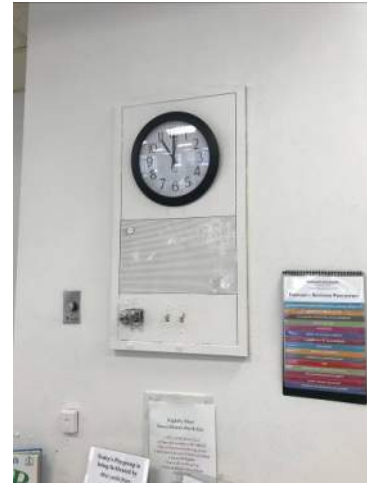
Classrooms Switches on C/S Panel
