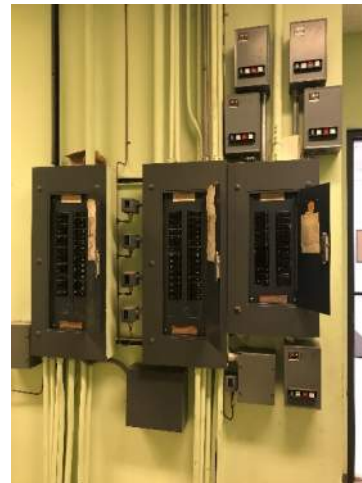
Panelboards on 3rd Floor
