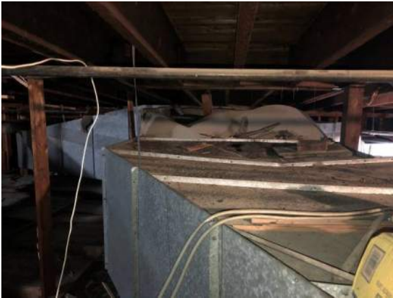
Attic – Exhaust/Ventilation Ductwork
