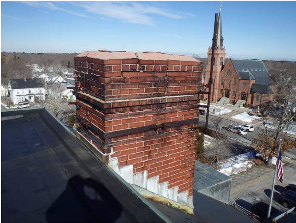
Figure 25. Northeast chimney showing open joints, cracks and iron straps
