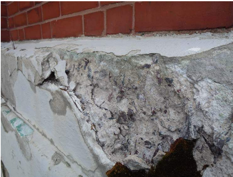
Figure 10. Deteriorated cast stone and purple aggregate (possibly rhyolite)
