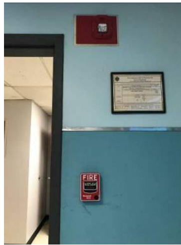
Pull Station & Horn/Strobe
