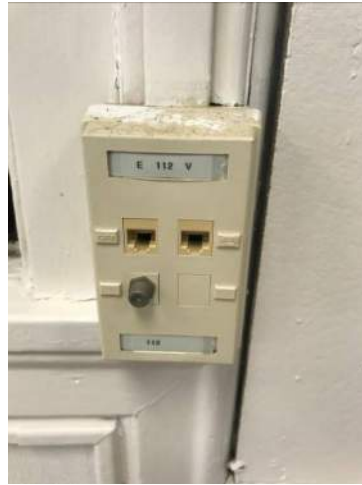
Data/Coaxial Outlet in Classrooms
