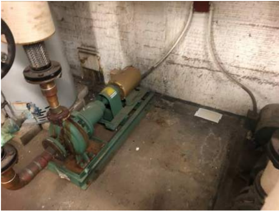
Existing Hot Water Pump P-4
