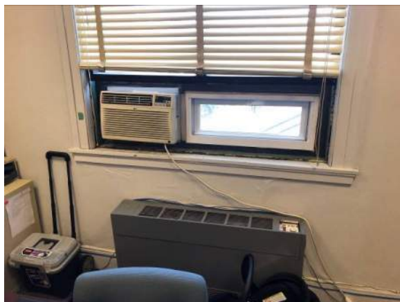
Administration Office – Window AC and HW Fan Coil
