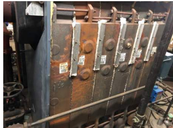
Existing Boiler - Cast Iron Sections
