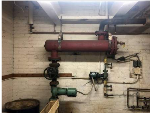
Abandoned in Place HW Heat Exchanger
