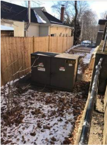
Pad Mounted Transformer
