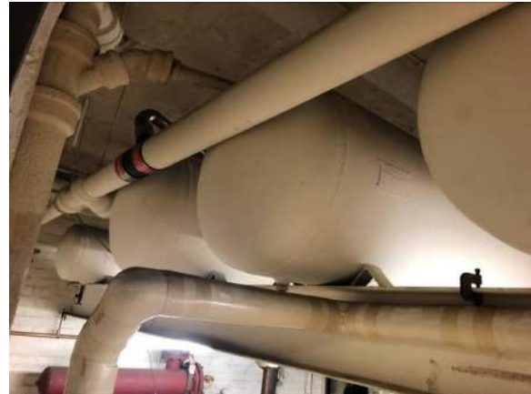
Abandoned in Place Expansion Tanks
