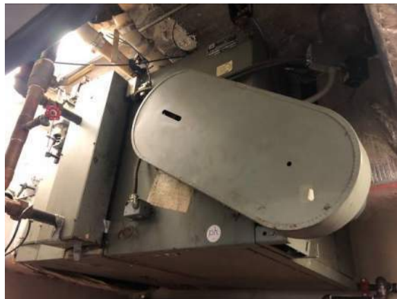
Kitchen/Cafeteria Heating & Ventilation Unit
