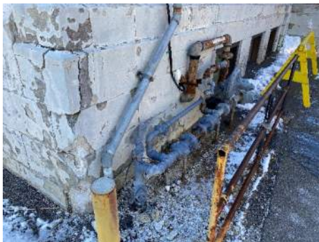
Building gas meter
