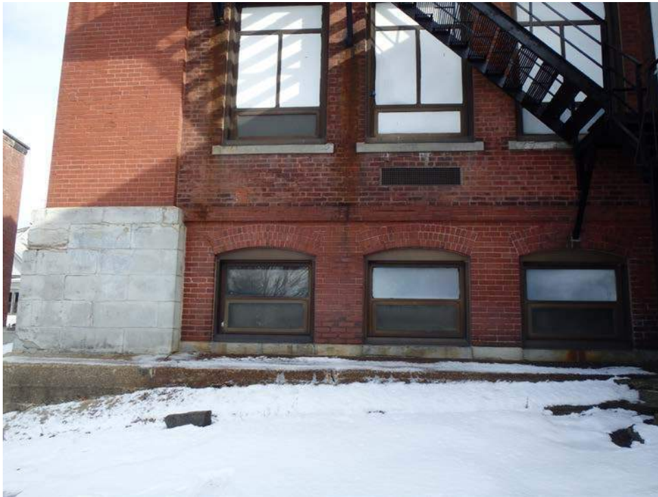
Figure 3. High quality brick used on north, south and east elevations (left) and lesser quality brick on west elevation (right)
