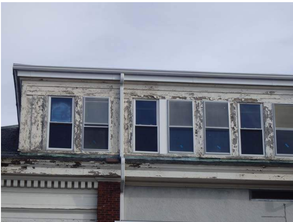
Figure 16. Paint failure and loss is extensive, exposing bare wood
