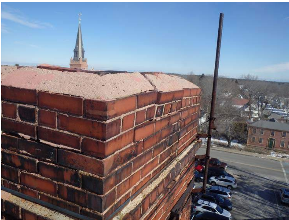
Figure 26. Northeast chimney – area of bulged brick at chimney top
