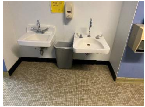
Typical wall hung lavatories
