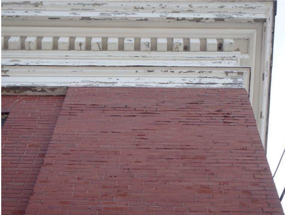
Figure 5. Area of failing and missing mortar joints
