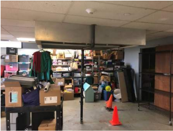
Kitchen Exhaust Hood
