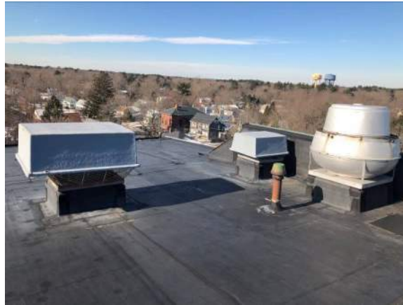
Roof - Exhaust Fans
