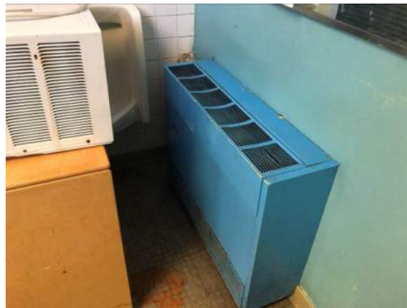
Toilet Room – Convactor Heater
