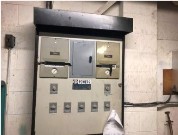
Existing ATC Pneumatic Control Panel
