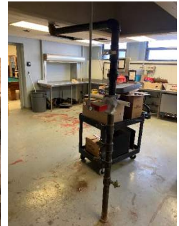
Natural gas piping in Kitchen
