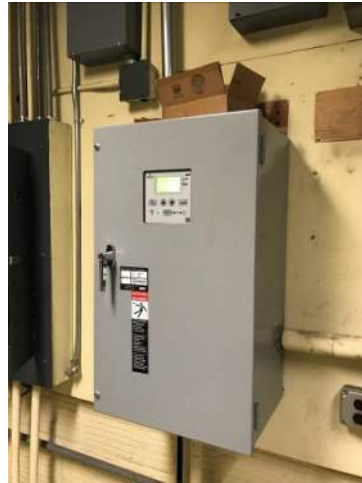
Automatic Transfer Switch
