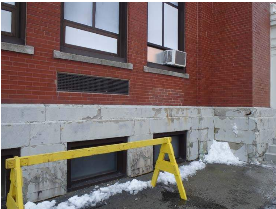
Figure 4. Area of brick infill with poorly matched brick and mortar
