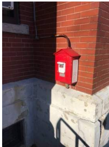
Exterior Master Box
