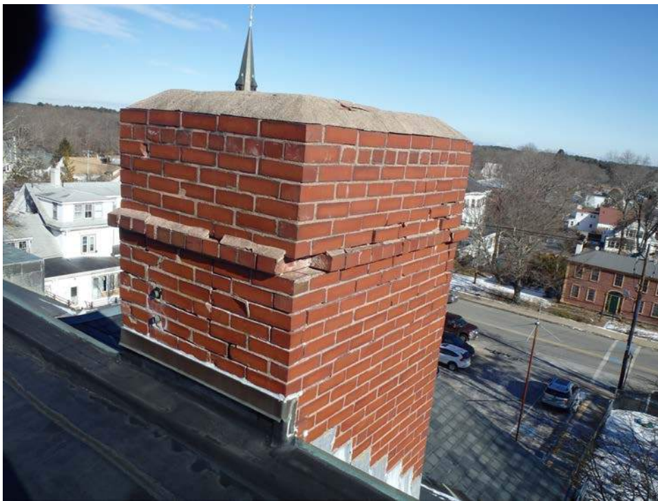
Figure 24. Southeast chimney showing missing brick and open joints
