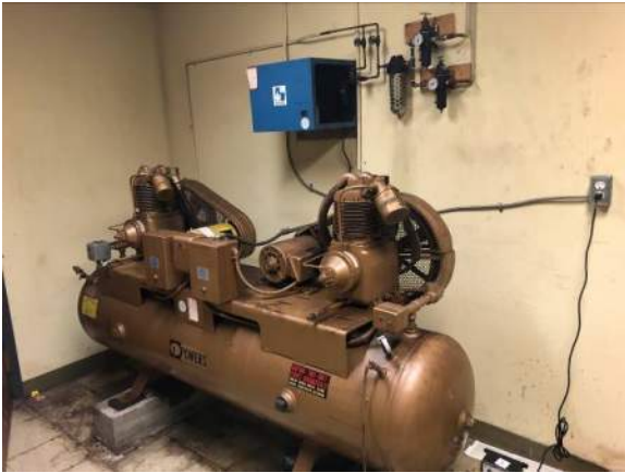
Existing ATC Compressor and Air Dryer
