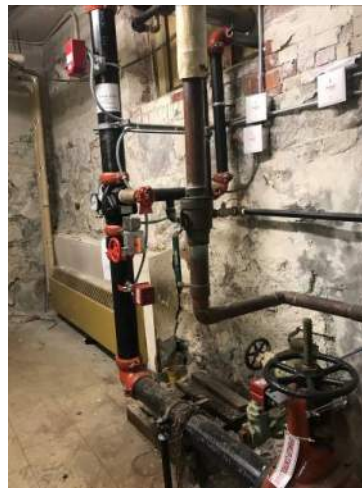
Sprinkler Flow & Tamper Switches
