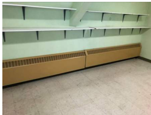
Third Floor Storage Room – Fin Tube Radiation
